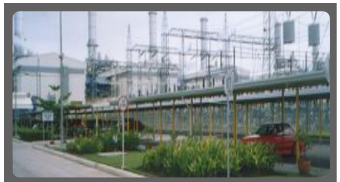
PIPE RACK AND PIPING
