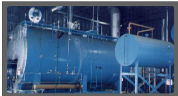
Blower / Tanks / Rollers
