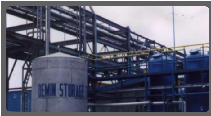
WATER TREATMENT PLANT PIPING
