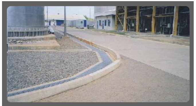
PLANT TRENCH GRATINGS
