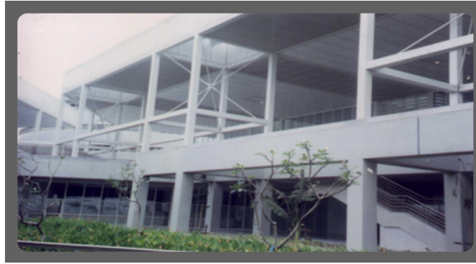
Fabrication of Steel Structure NAIA II Terminal LKS DEVELOPMENT CORP. Canlubang Industrial State, Laguna
