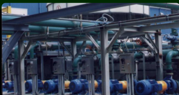
Rollers, Steering Units and Pumps
